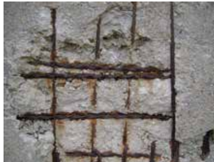
Spalling From Concrete Cancer
