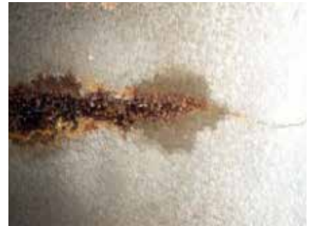
In-Situ Corrosion of Steel Reinforcement
